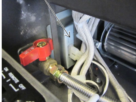
Junction Box (from inside fireplace)
