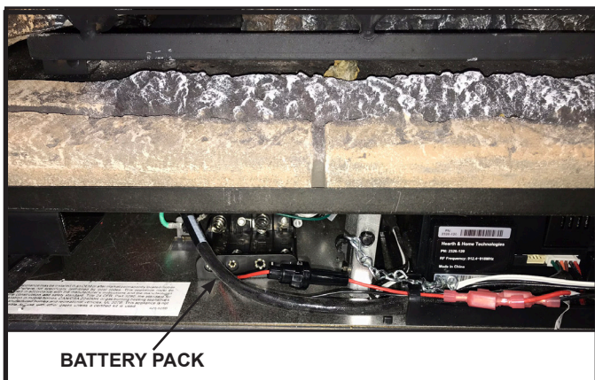
Figure 3.8 Battery Pack Installed
